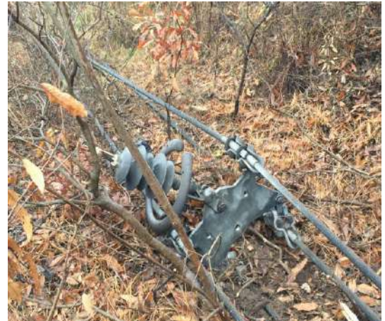
Figure 2 The wire has fallen to the ground.
